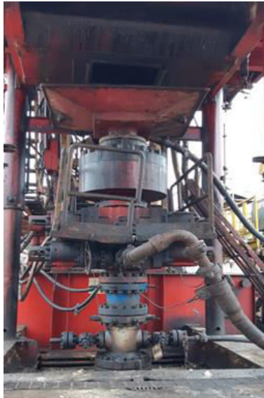
Fig.17. Pilot Project of The BOP Side Outlet Usage in a 11" Class III BOP Stack (Source: Internal documentation)
